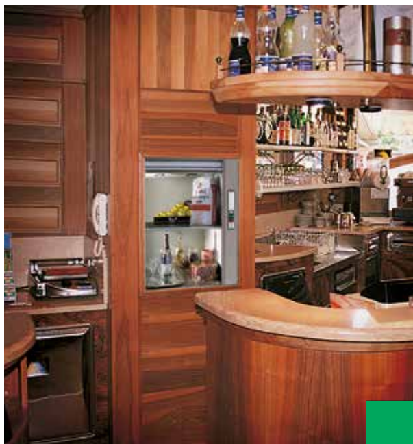
Installation in a restaurant-bar (Italy), model 50 kg with wood cladding. It perfectly fits the environment.
